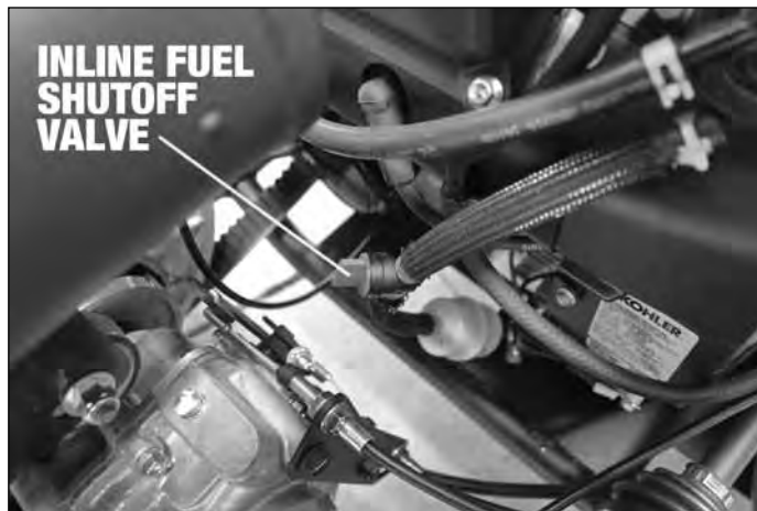
figure 4.19 (inline fuel shutoff valve shown in the "ON" position)
